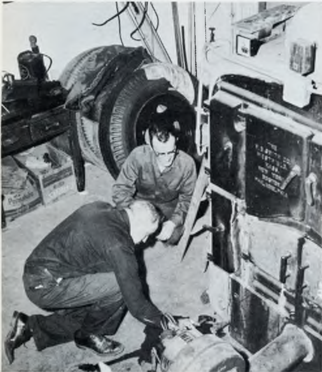
Fred Clark and Paul Rumley check boiler in Community Center
